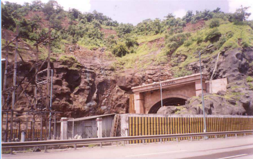
DEBRIS FLOW AND ROCKFALL
