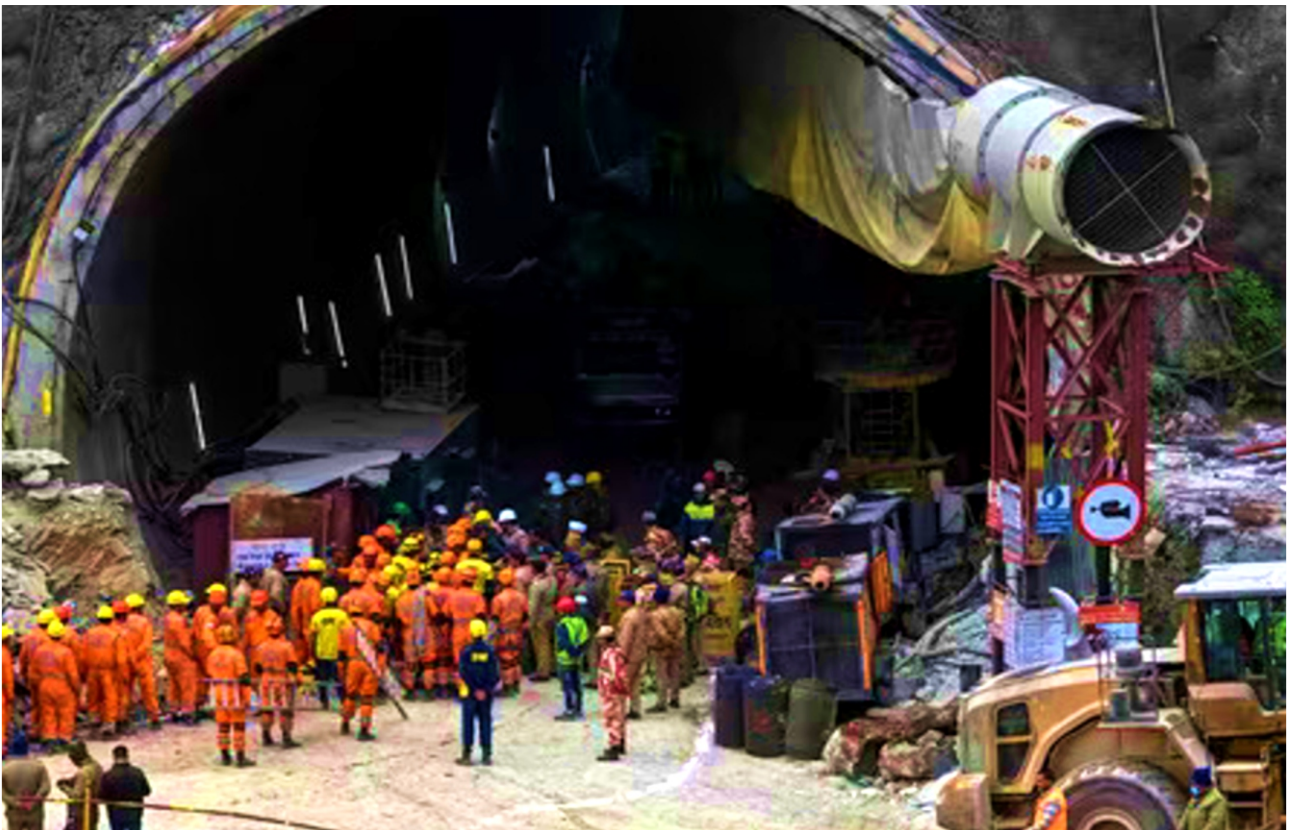
Photo 1: Photo taken during rescue operation at Silkyara Tunnel during Nov. 2023. Source: Pic Credit: Hindustan Times
