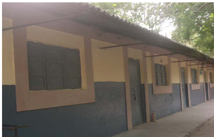
Fig.5 :- Seismic belts provided in a school building at ceiling level and around openings
